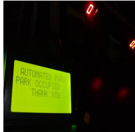
Figure 10: LCD display showing that the parking lot is fully occupied
