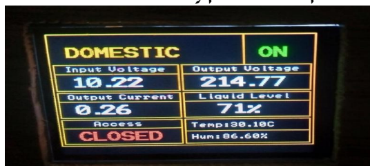
Fig. 6: TFT LCD Screen Result Showing Transformer Parameter
