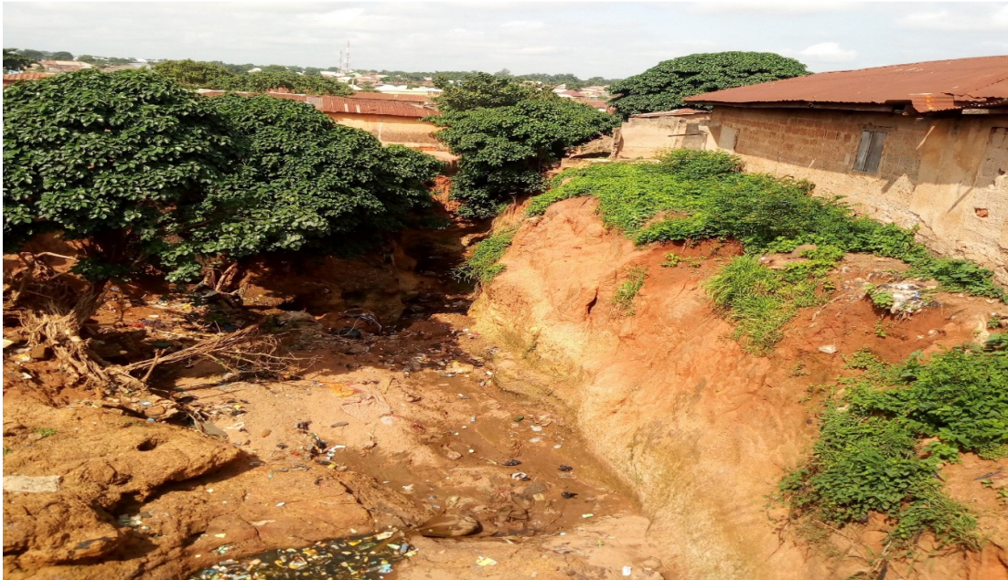
Plate 5: A typical gully cross-section in Gimare, Lafia LGA
