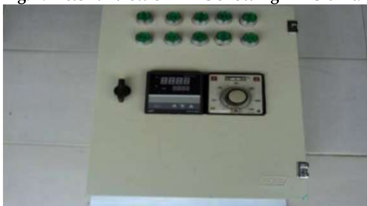
Fig. 2: Control panel with two temperature controllers and ten normally-open push buttons.
