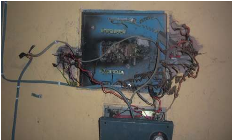
Fig 1: Faulty load distribution on the distribution board
