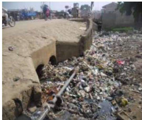
Wastes dumped inside culvert in Unguwar Gade food in gwagwalada abattoir.
