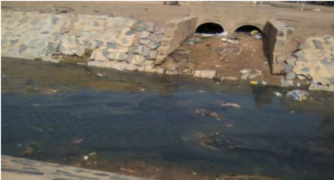
Figure 4.6: Blockage drainage at Limawa ward
