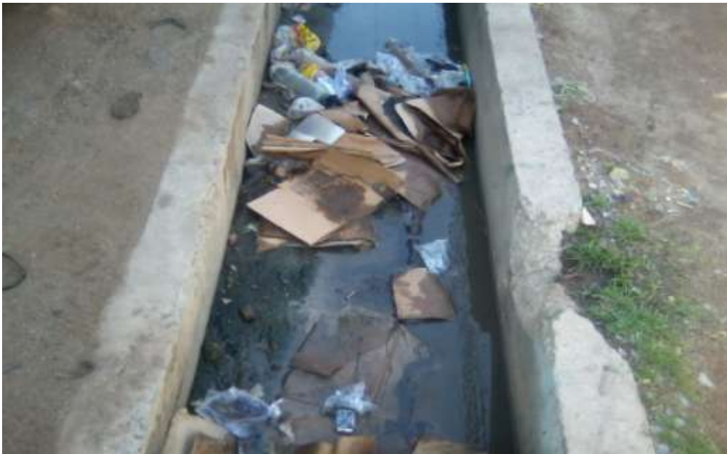
Figure 4.5: Blockage drainage at Rumde ward
