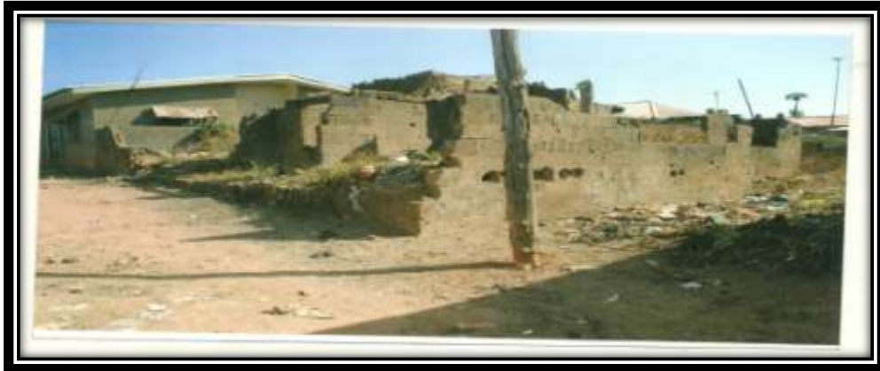
Plate 6: Uncompleted Building Converted As Refuse Ground within the Residential Area of Mararaba Gurku Area of Nasarawa State
