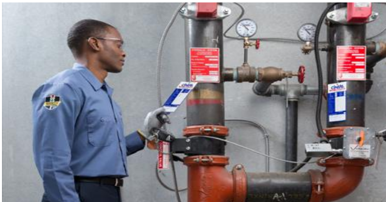
Plate 1: Fire Sprinkler System [Source: Cintas Corporation, 2016 ( http://www.cintas.com/fire-protection-services/fire-sprinkler-systems.aspx )].
