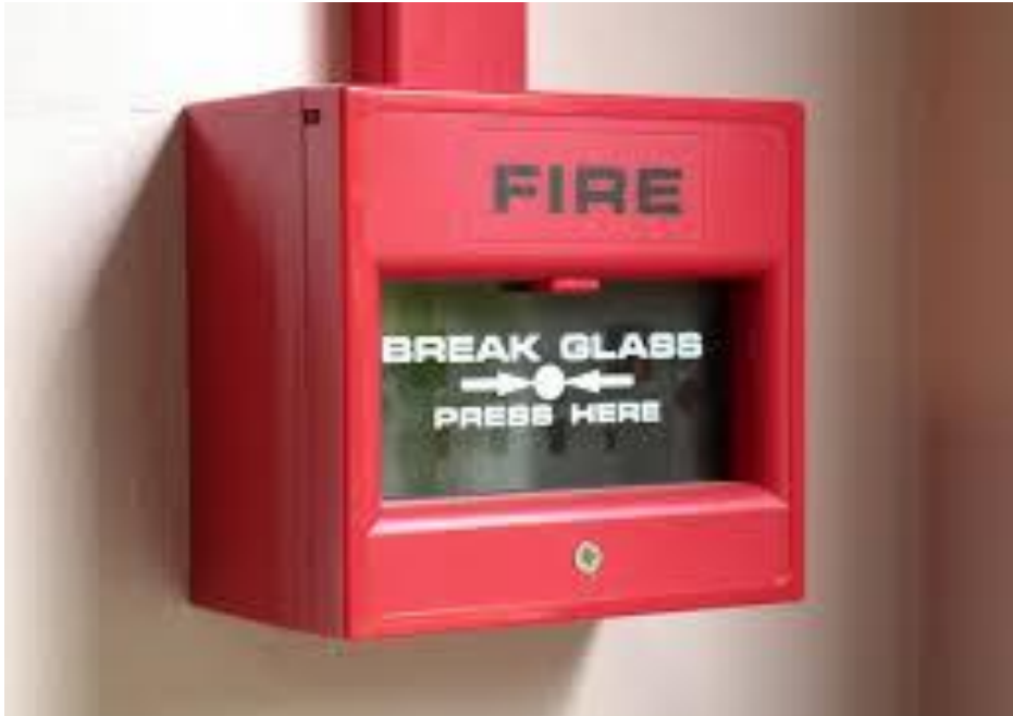
Plate XII: Fire Alarm [Source:WELT Limited, 2013 ( http://weltuk.com/FIRE-ALARMS )].
