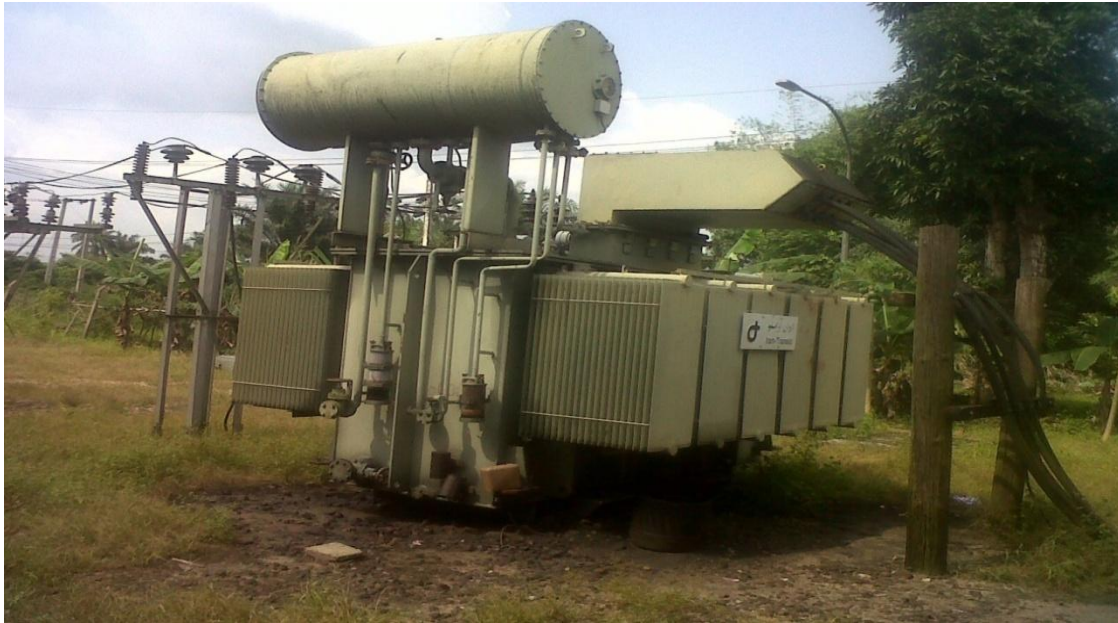
Figure 1: Photo View of U-15, 15MVA, 33/11kV Injection Substation.
