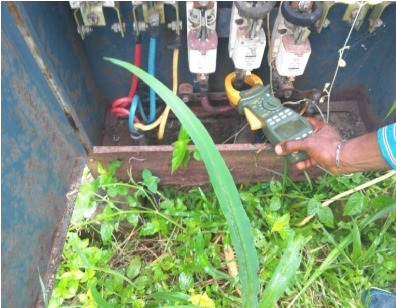
Fig. 3. Reading being taken from a Substation Feeder Pillar.
