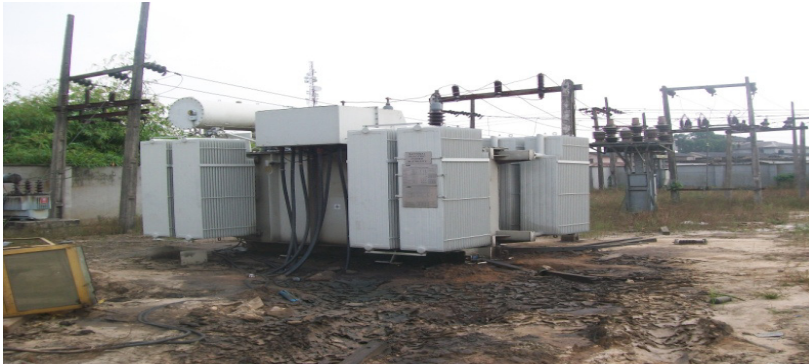
Fig. 2 Photo view of Otovwodo, 15MVA, 33/11KV Transformer.
